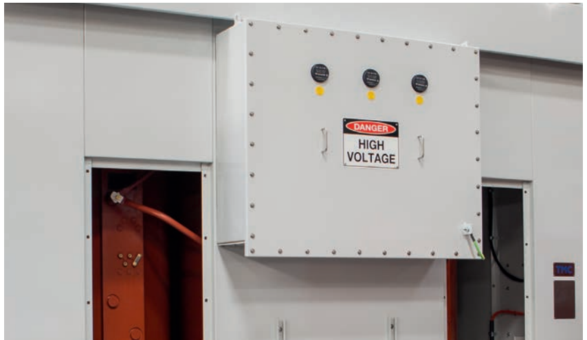
IP 43 (doors removed) showing Cable Box and front panel with infrared thermographic inspection windows
