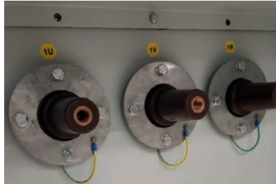
HV Cable Box with Separable Connectors
