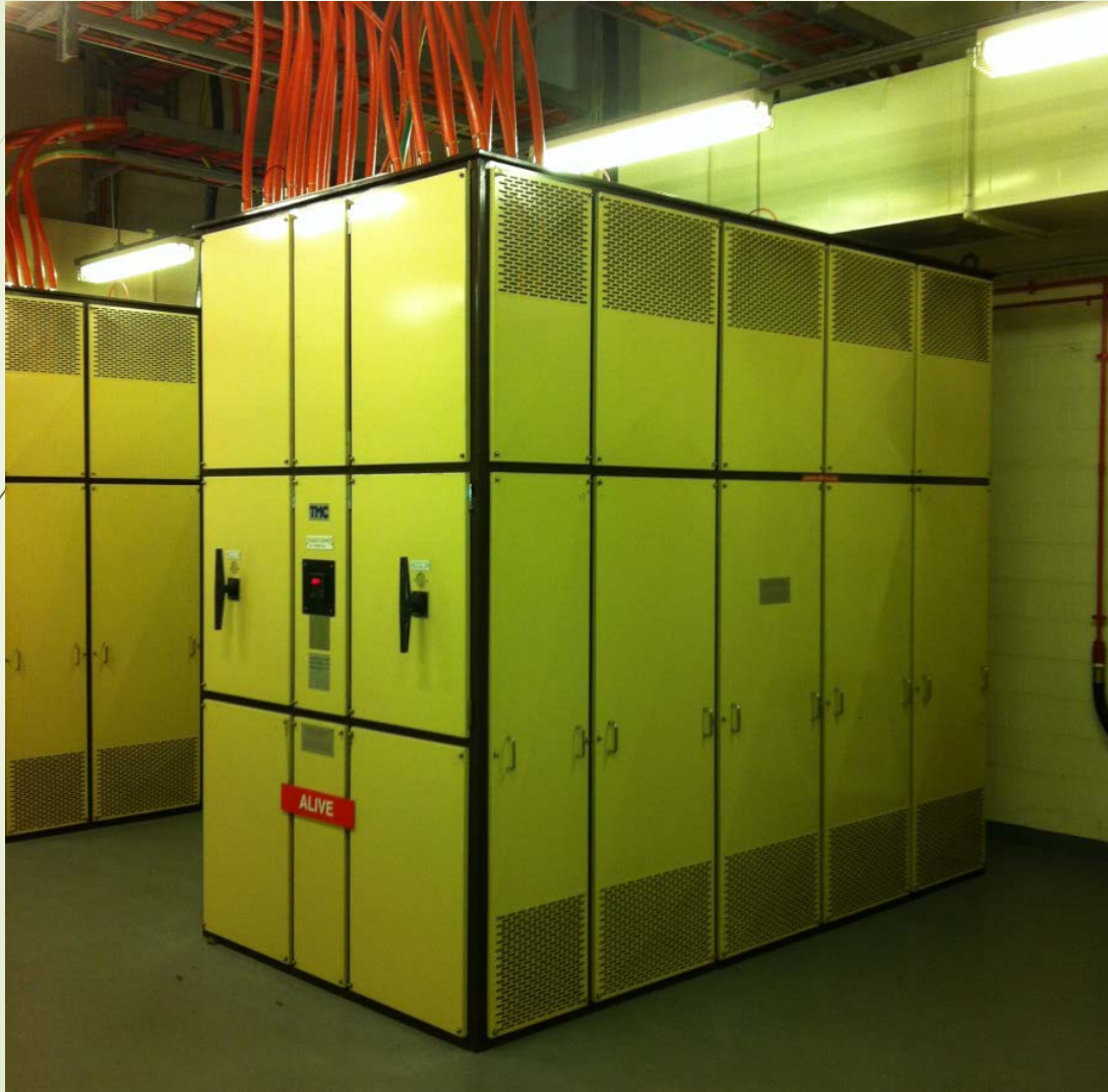
2000kVA 22000/433V Cast Resin Transformer, AN IP21 Data Centre
