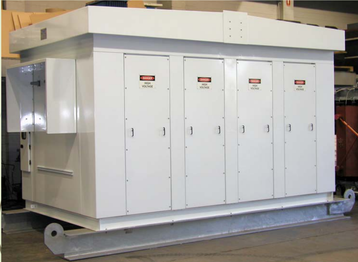
4MVAr 33kV Capacitor Bank with 41.3mH 33kV 75A Filter Reactor , AN IP43
