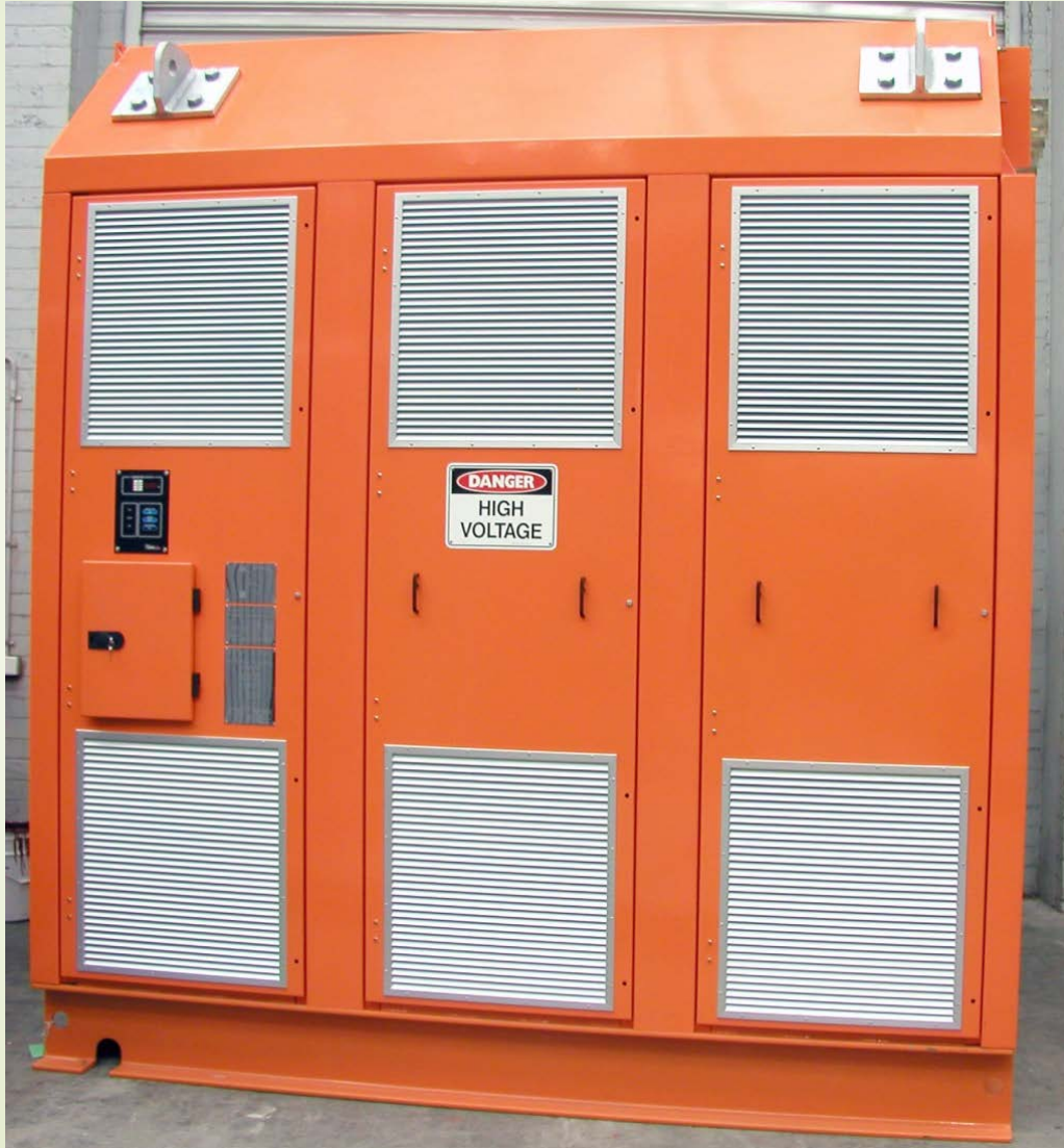
3000kVA 11000-6600/600-600V Cast Resin Transformer, AN IP43
