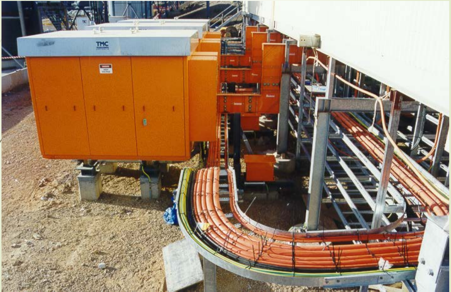
2000kVA 11000/690V Cast Resin Transformer, AN IP43 Material Handling Plant
