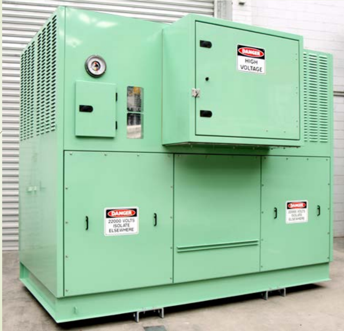
2800kVA 22000/1700-1700V Cast Resin Transformer, AN IP21 1 of 12 in a 144 Pulse System
