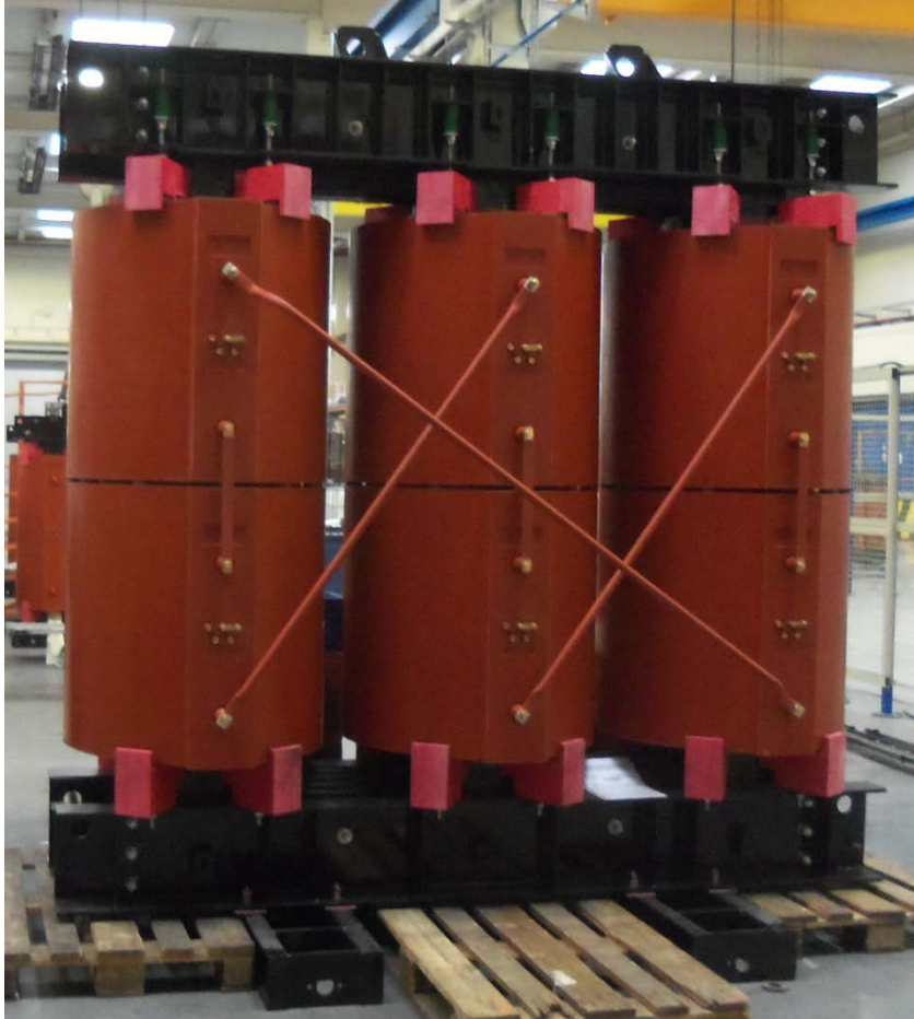
TRANSFORMER 4 MVA 21/6,3 KV
